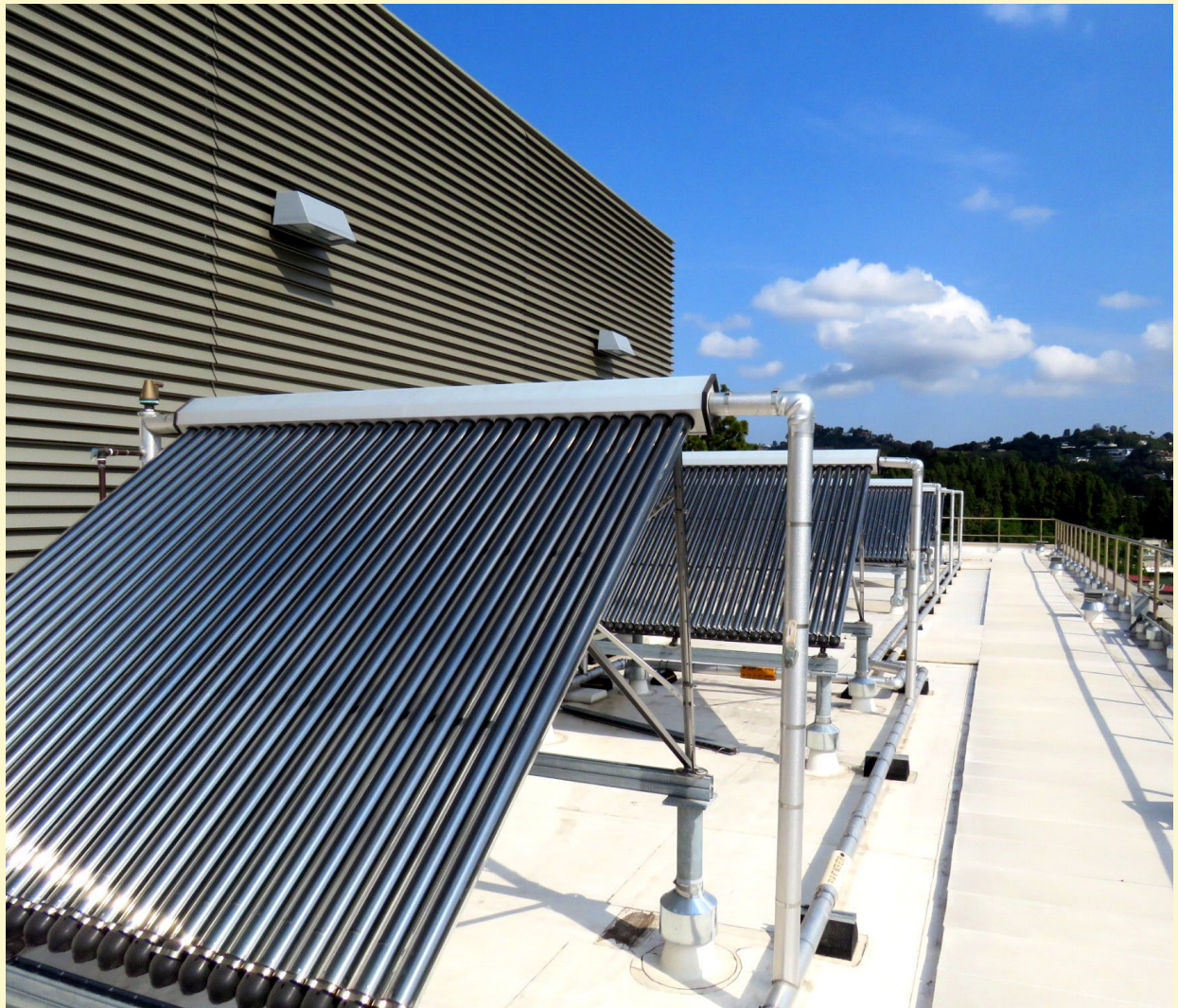
Evacuated tube solar water heating installation at UCLA's residence halls.
