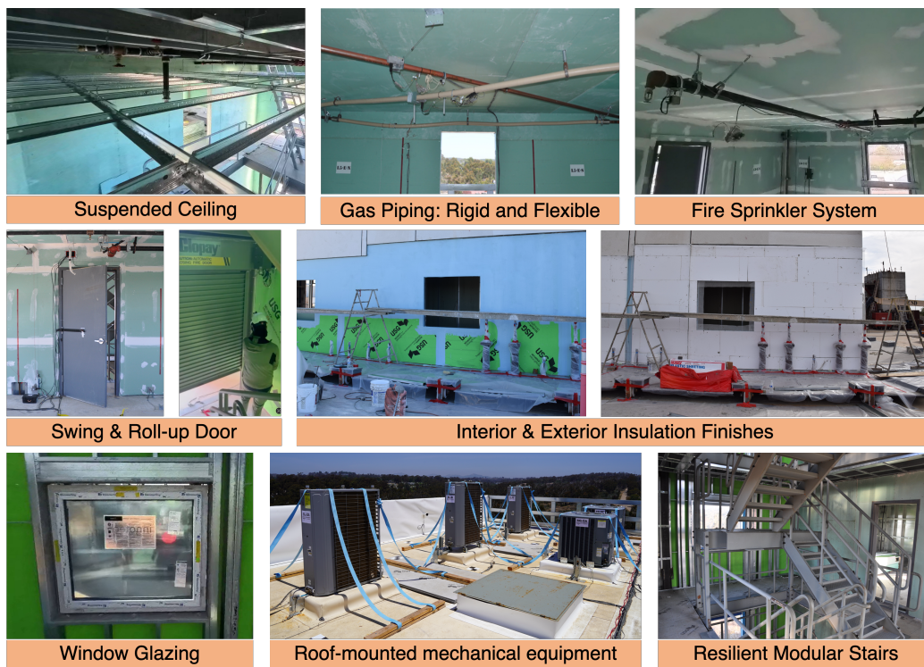
Figure 2. Nonstructural components and systems installed in the CFS10 building.
