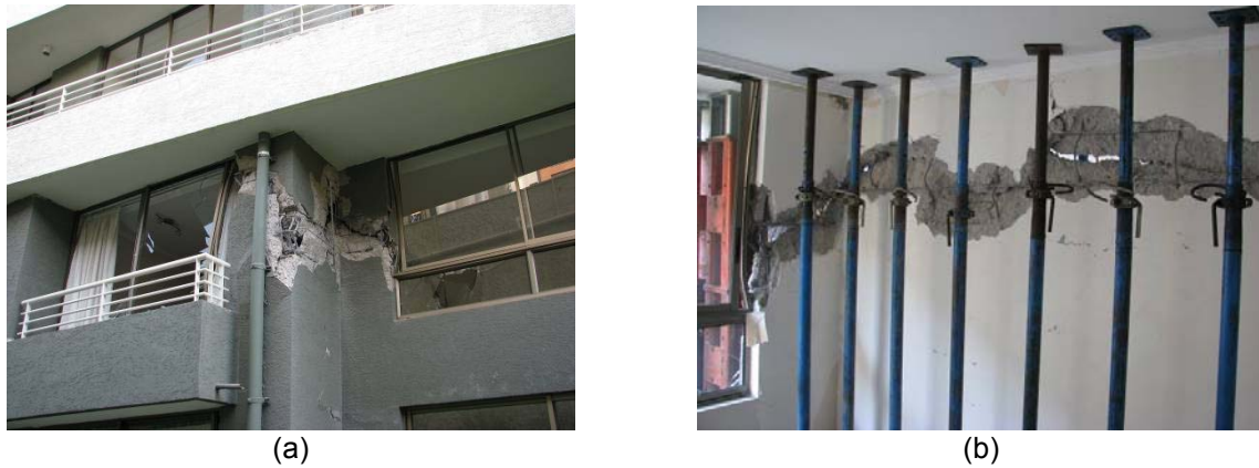
Figure 6.54 Damaged walls in second story, axis J: (a) view 1; (b) view 2 (after DICTUC, 2010).
