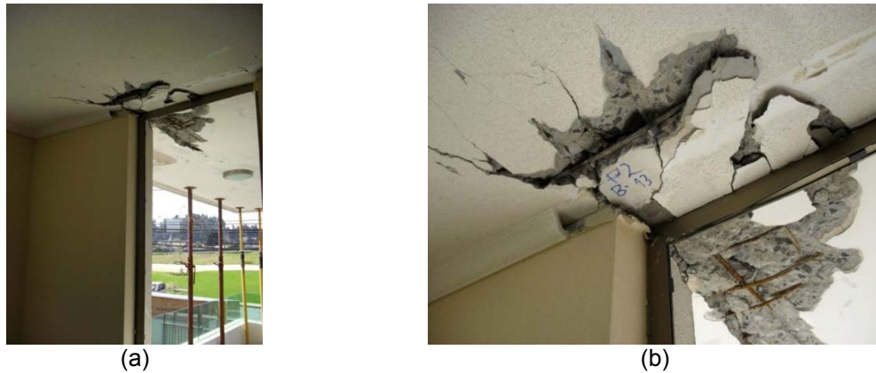
Figure 6.18 Second story damage in axis C, between 13 and 14: (a) view 1; (b) view 2 (after DICTUC, 2010).
