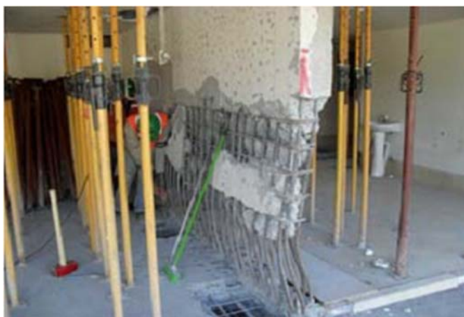
Figure 1.1 Buckled wall in first story of Building #1 (DICTUC, 2010).
