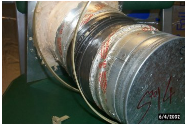
Figure 12. The failed plastic strapping on one of the flexible core to sheet metal collar specimens after four months of aging.
