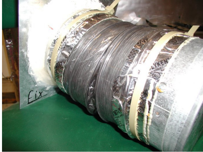
Figure 11. Oozing of the adhesive layer in the foil-butyl tape (Tape 4) specimens (showing result of 5 months of aging).
