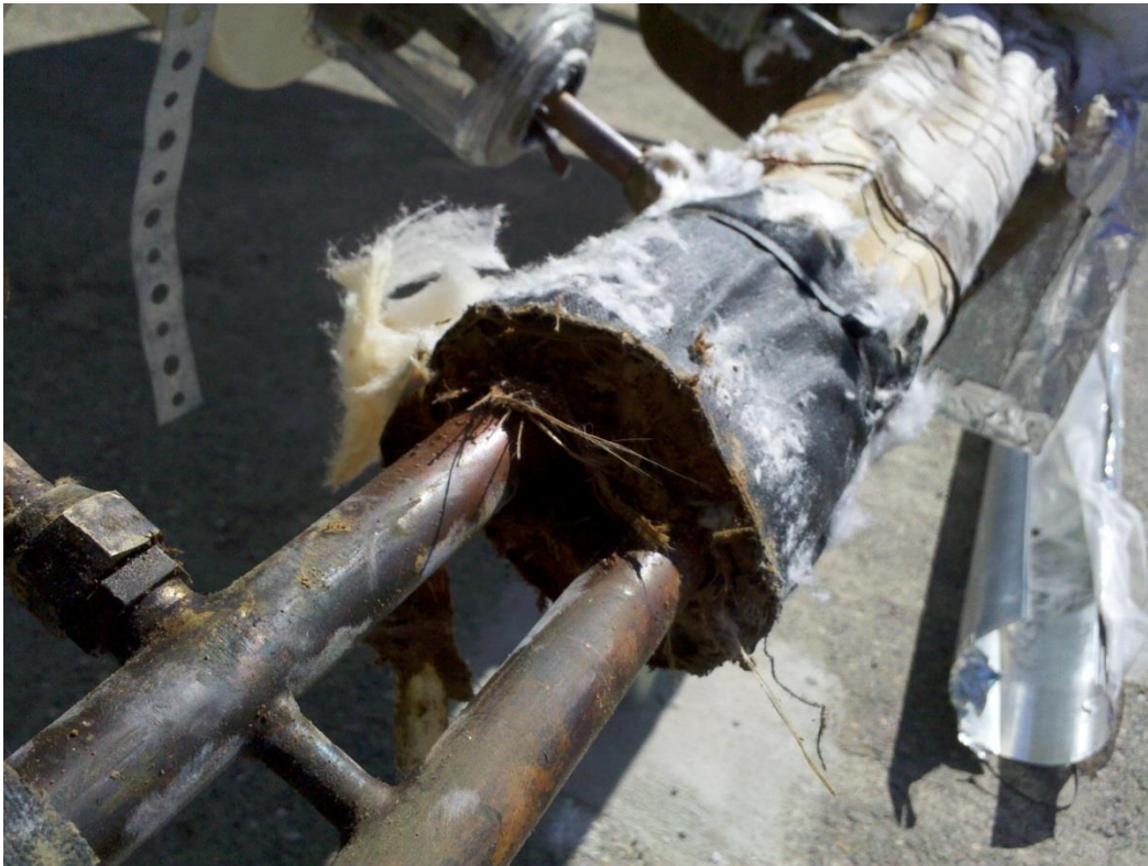
Figure 28 – Insulation damage from oil leaks
