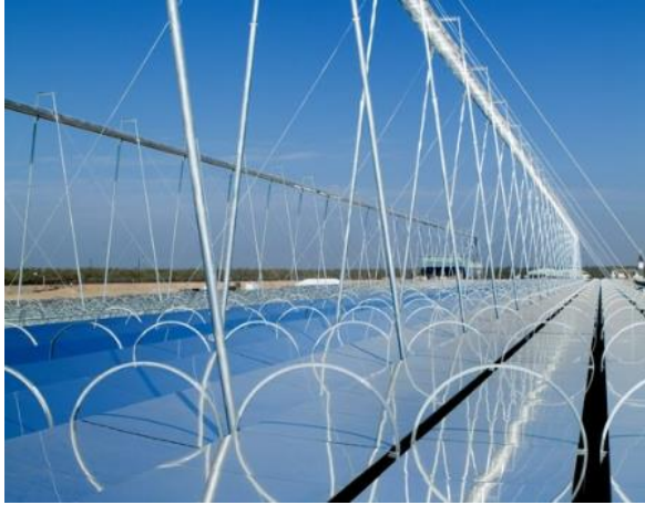
Figure 5 – Linear Fresnel Solar Plant
