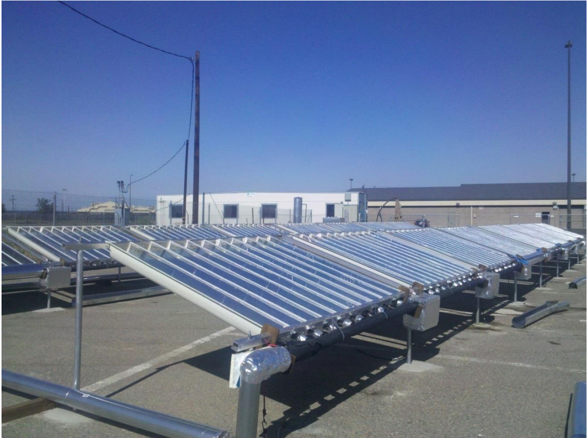
Figure 34 – XCPC array at UC Merced Castle research facility
