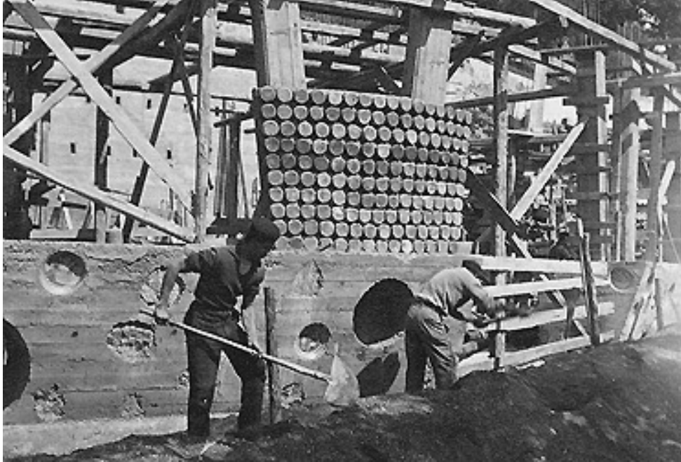
Figure 7. Construction of the Ceramica Solimene, where company ceramicists made the cylinders that clad the spiral-ramp factory. 1952. Paolo Soleri Archives, Cordes Junction.
