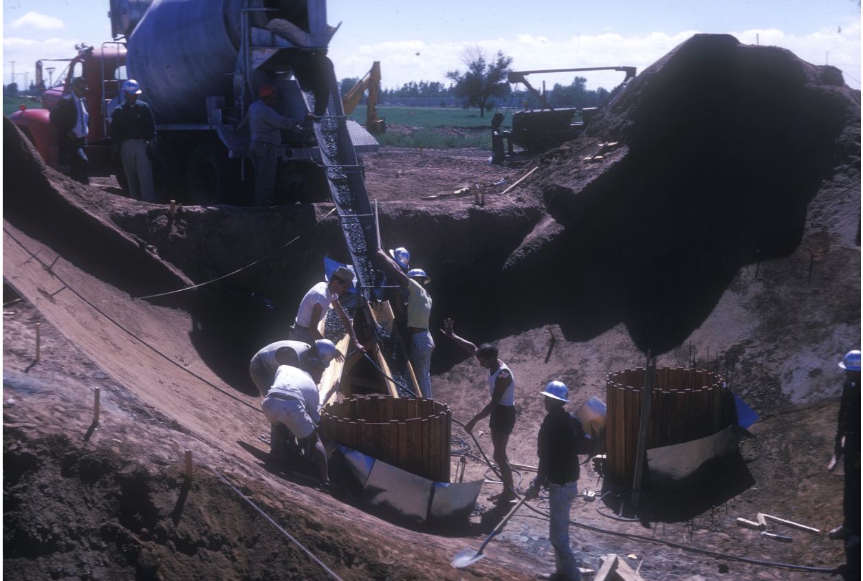
Figure 24. Soleri, Colly. Photograph of Soleri with apprentices and students on first pour. Santa Fe. June 1966. Paolo Soleri Archives, Cordes Junction.
