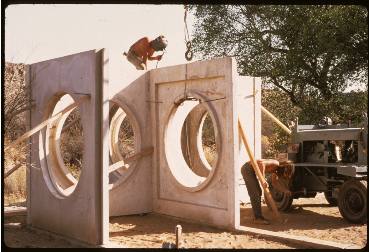
Figure 33. Annette Del Zoppo. Photo of volunteers constructing sleeping cubes for camping, 1972. Paolo Soleri Archives, Cordes Junction.
