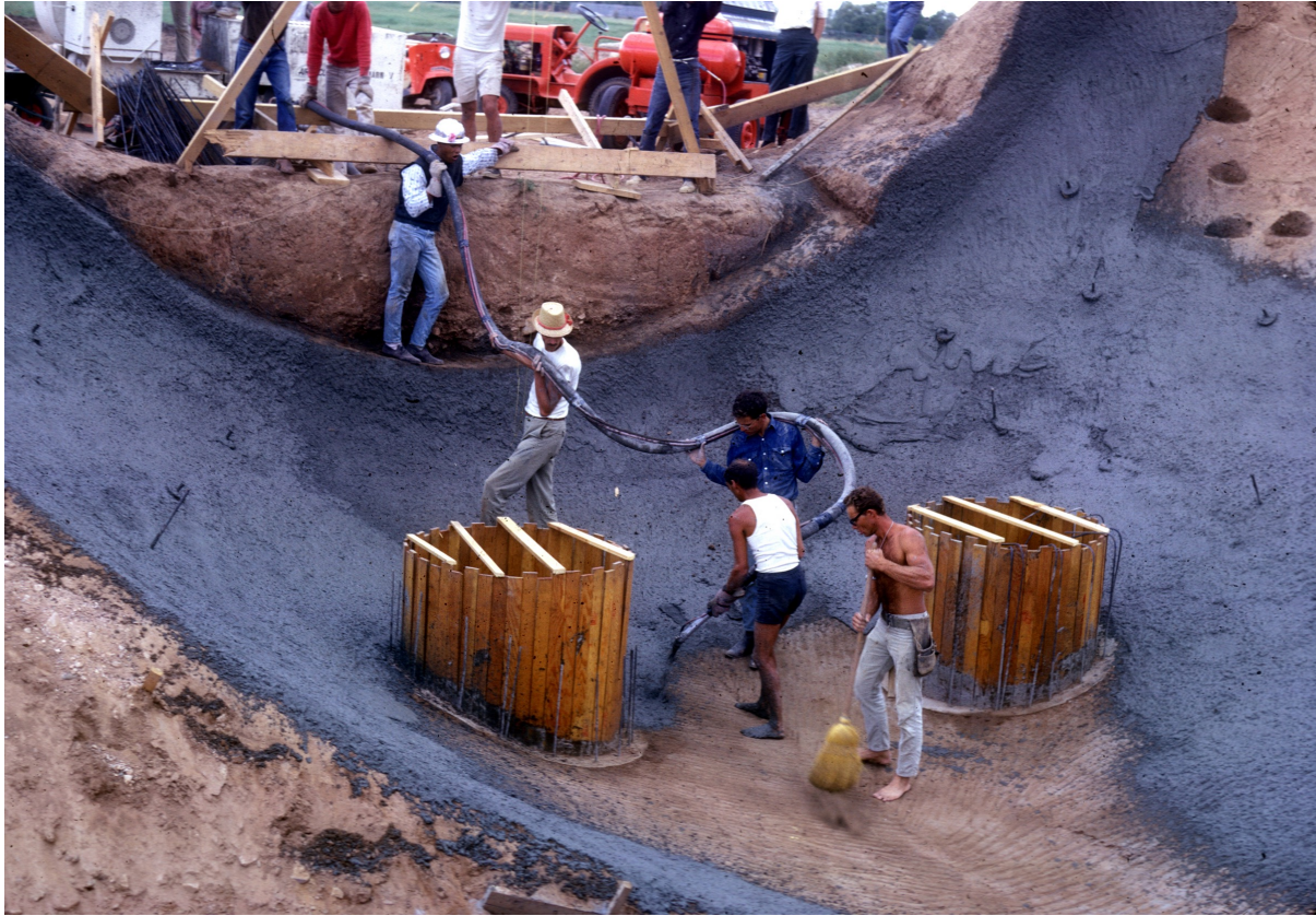
Figure 25. Soleri, Colly. Concrete pour on IAIA amphitheater. Santa Fe. June 1966. Paolo Soleri Archives, Cordes Junction.
