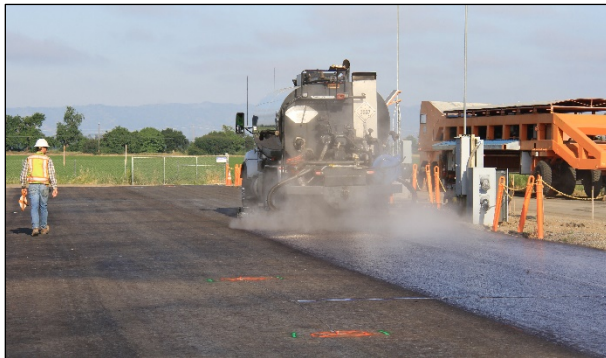
Figure 4.31: RHMA-G: Tack coat application before first lift of RHMA-G (Cells H and I).
