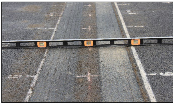
Figure 9.18: 701HC: View of rut at Station 8.
