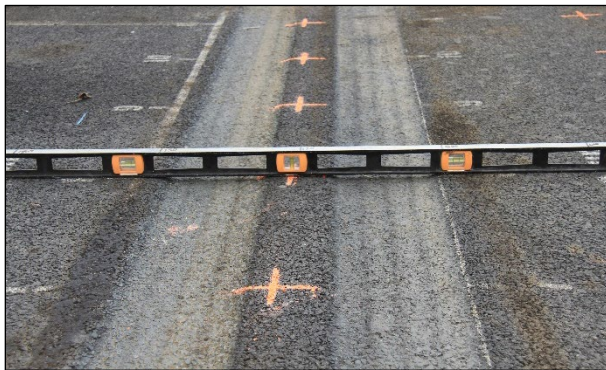
Figure 7.18: 704HB: View of rut at Station 8.
