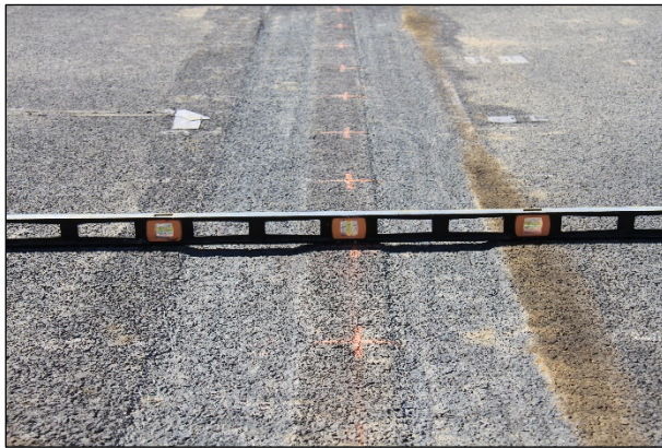
Figure 8.16: 703HB: View of rut at Station 8.
