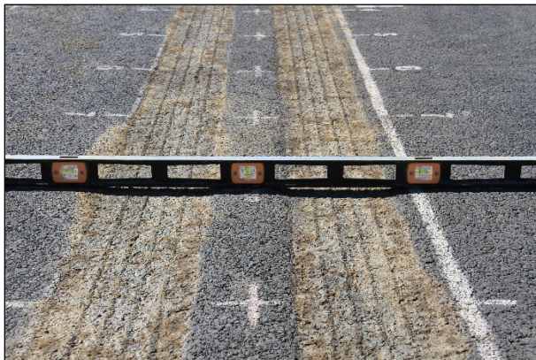
Figure 10.20: 698HC: View of rut at Station 8.
