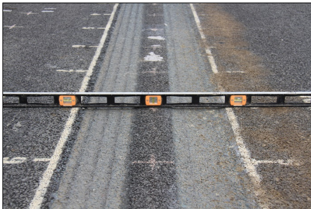
Figure 11.18: 700HB: View of rut at Station 8.
