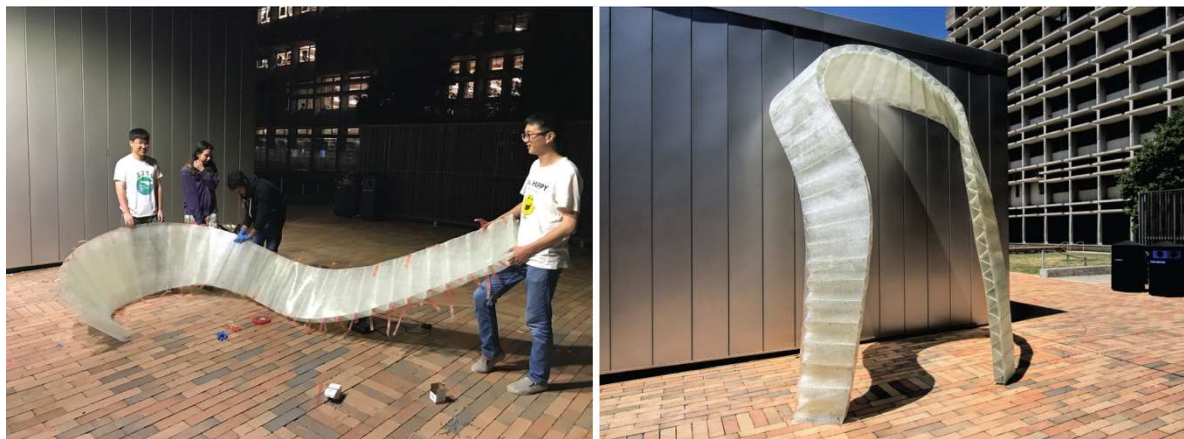
Figure 19. Students assemble the 8-m-long, curved sandwich strip of the pavilion in full scale.
