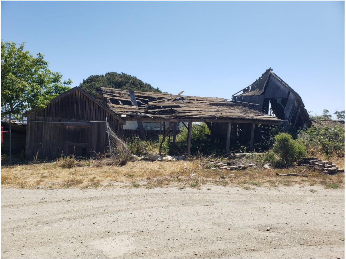
Figure 8.22. Collapsed Hirahara Carriage Barn photographed by author June 6 th , 2021.
