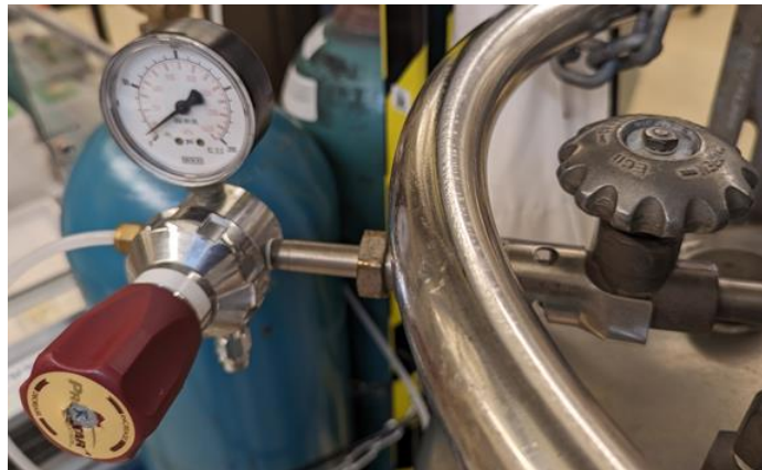
Figure GA.4.14. Liquid Ar valves. The tank open/close valve is on the right.
