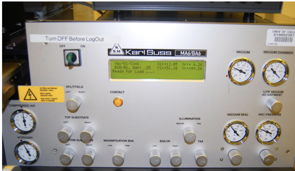
Figure 3.31: MA6 control panel.
