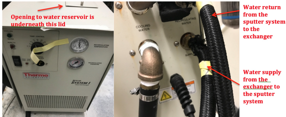
Figure A.20: Heat exchanger front (left) and back (right)
