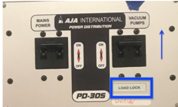
Figure A.5: Controller for load-lock pump and power- turn the vacuum pump switch on to pump down the load-lock.
