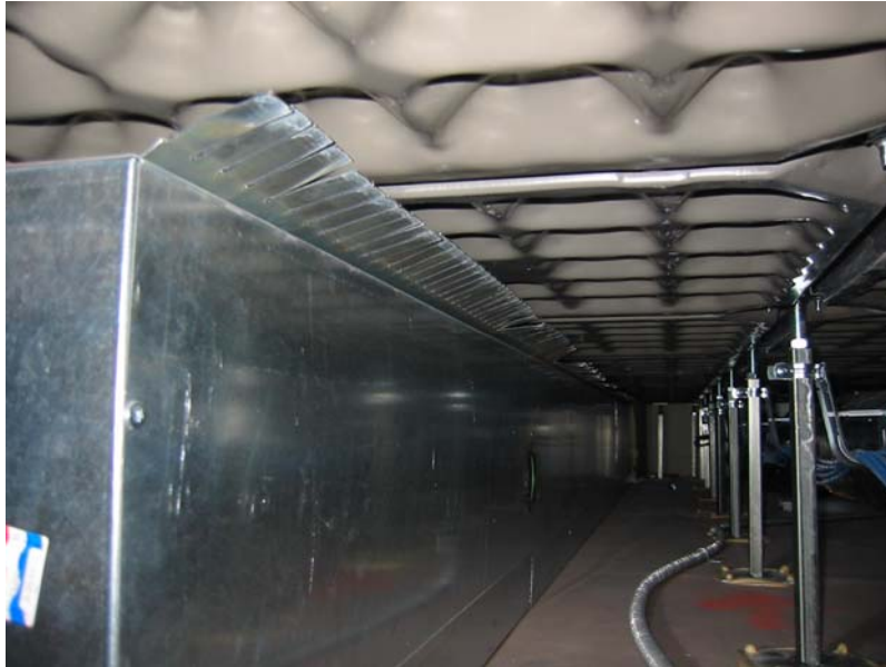
Figure 11. Installation of Acoustical Septum. The metal fingers at the top of the septum were later pushed into floor panel coffers, forming an acoustical seal at the septum and floor panel.
