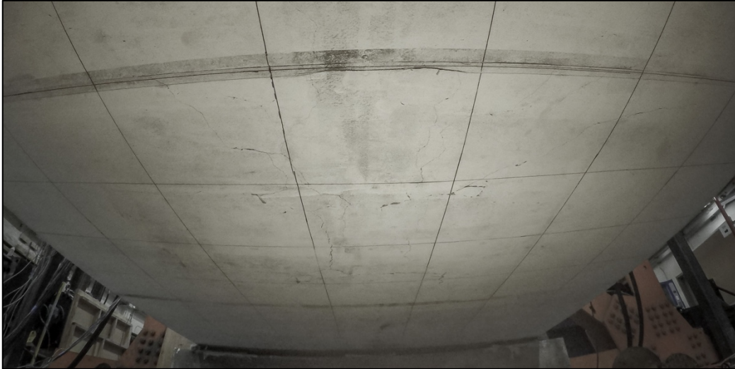
Figure 5-6. Damage observed on the bottom surface of the specimen after failure as seen from east to west
