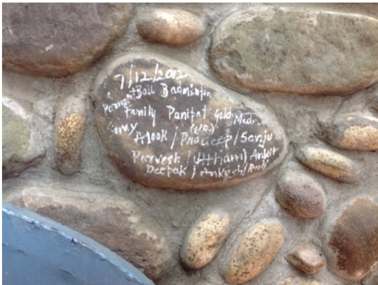
Figure 51: Graffiti on wall into Phase III [photograph by the author, 2014]
