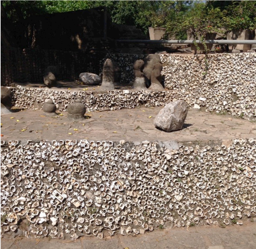
Figure 37: Wall surfaces clad with fragments of electrical moldings [photograph by the author, 2014]
