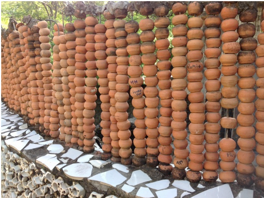
Figure 81: Wall constructed of terracotta pottery, broken tiles, and fixtures, Phase I [photograph by the author, 2014]
