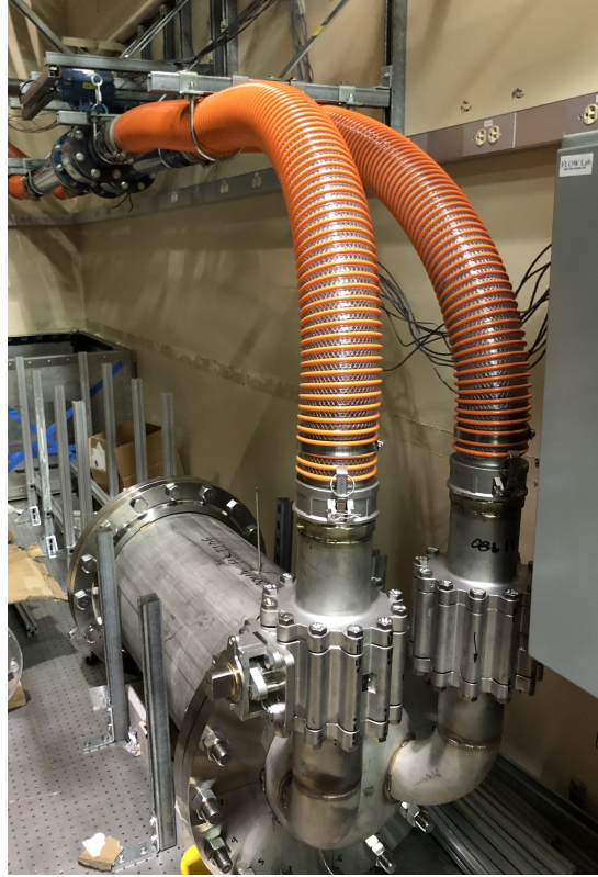
Figure 3.8: The assembled contraction tank includes two 102 mm (4" nominal) ball valves used to isolate the upper section of the flow loop during system priming.
