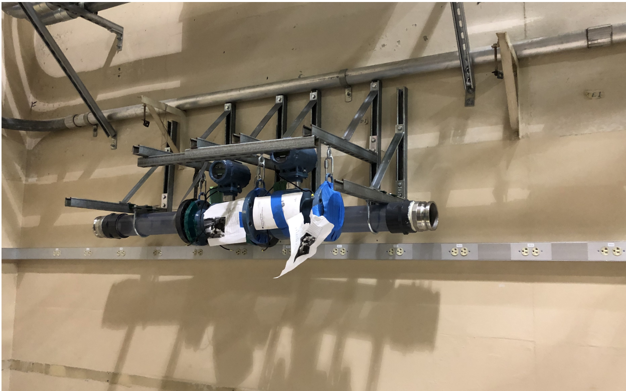
Figure 3.4: The magnetic flow meters are mounted horizontally, cantilevered from the wall above the optical table.
