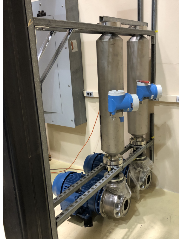
Figure 3.3: The Coriolis flow meters are mounted vertically in line with the outlet of the pumps.
