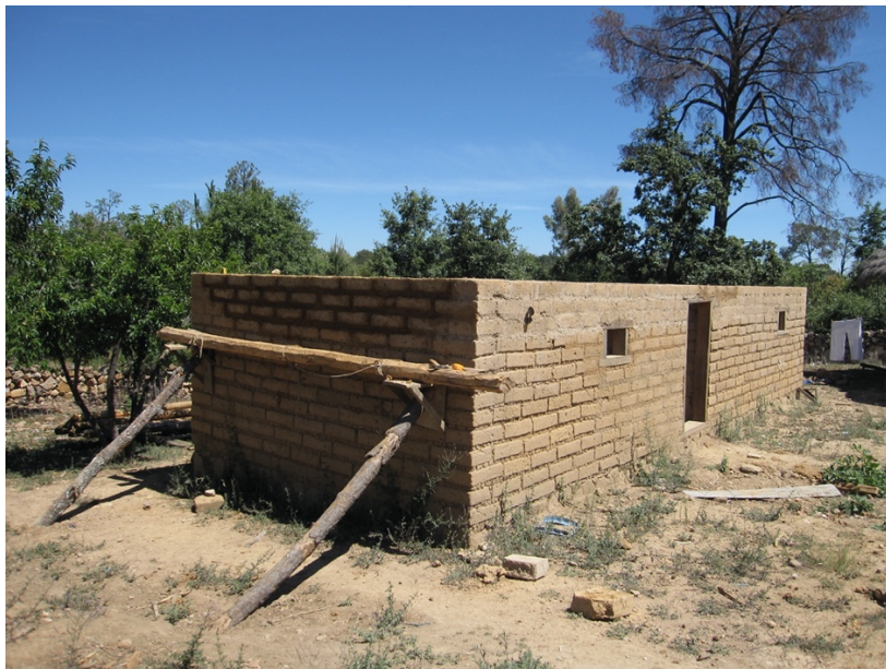
The walls are complete in this picture. The next step was the roof.
