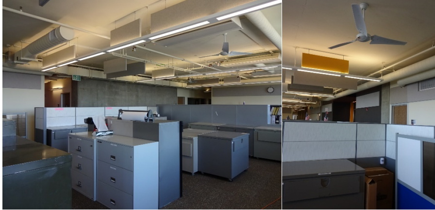
Figure 5-9: Typical open plan office space with TABS radiant ceiling, ventilation ducts, acoustical baffles, and ceiling fans.
