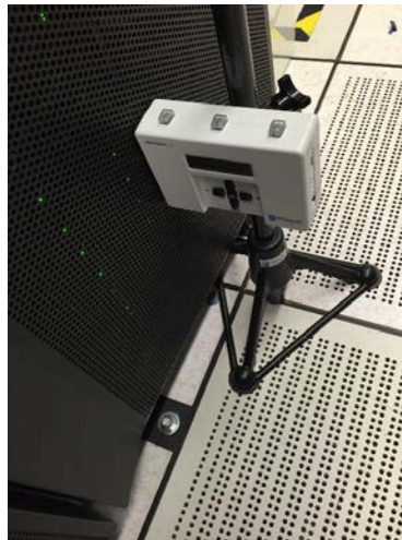
Figure 18. PurkeyLabs: No obstruction. Units can be placed close to the rack fronts.
