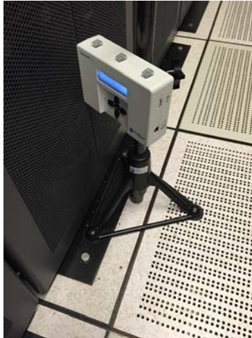
Figure 17. PurkeyLabs: Seismic bracing. Units cannot be placed close to the rack fronts.
