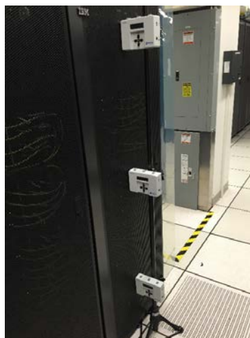
Figure 16. PurkayLabs: System fully assembled outside of rack R-29.
