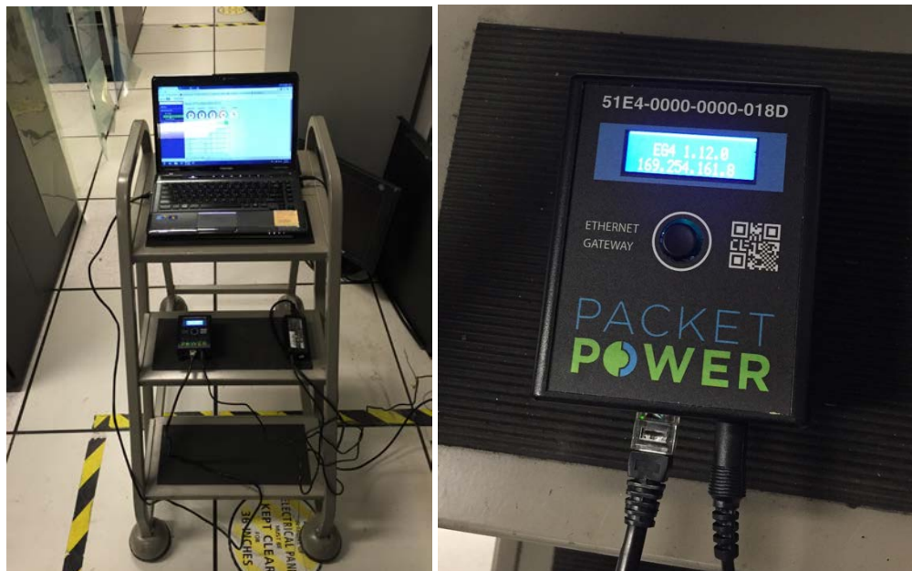
Figure 9: Packet Power: Gateway-4 (middle shelf – detail at right) and laptop. Gateway-4 connects wirelessly to E302. Laptop shows the Ethernet Gateway Console with temperature data.
