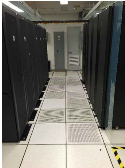
Figure 2. Aisle Layout. Rack R-26 is in the left foreground; R-29 is in the right foreground.
