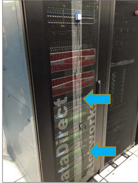
Figure 8: Packet Power: System installed on equipment rack. The blue/white box on the upper part of the rack door is the E302 unit. The two external probes are hanging down along the door (at arrows).
