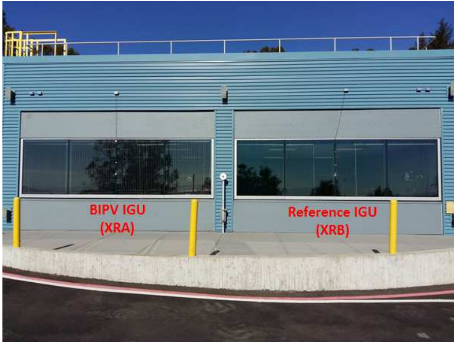
Figure 6 Picture of the BIPV IGU and the reference IGU installed on the XR rotatable test bed
