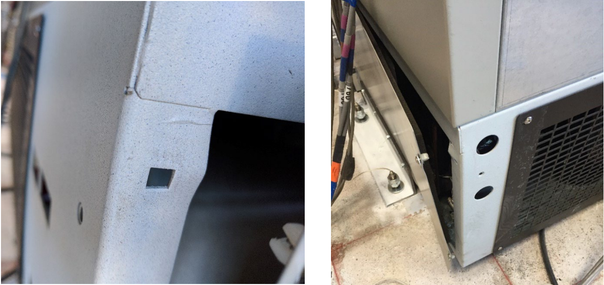
Figure 19. Freezer base after local failure at the two locations in the frame
