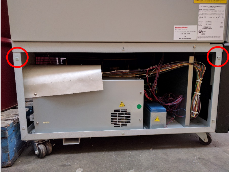
Figure 18. Freezer base with the location of the failures
