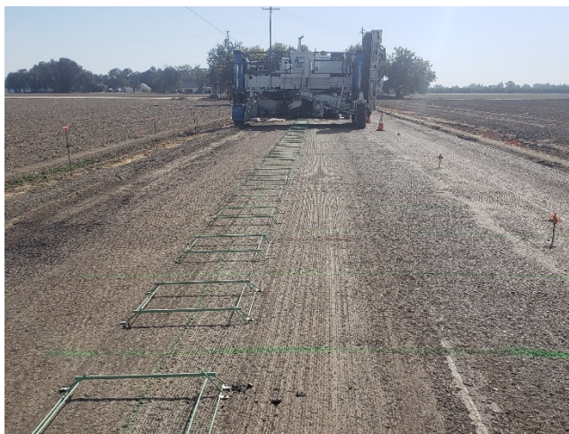
Compliant tie bar baskets
