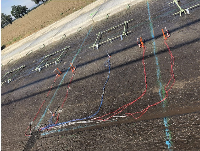
All sensors fixed to rods or chairs, zip ties tips and sensor labels cut, cables fixed with epoxy to the asphalt base.
