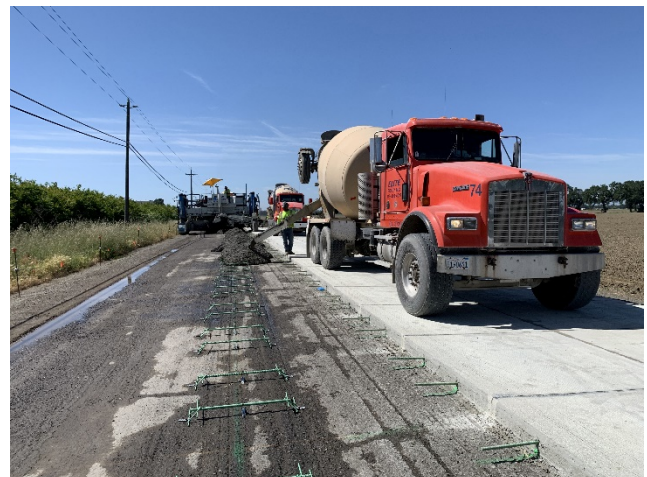
Asphalt surface is not adequately wet conditioned: some dry areas; standing water at the shoulder
