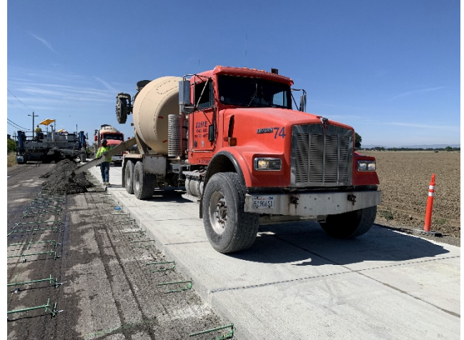
Occasionally, the ready-mix trucks discharged concrete directly on the lane, then the spreader spread the concrete over the width of the lane.
