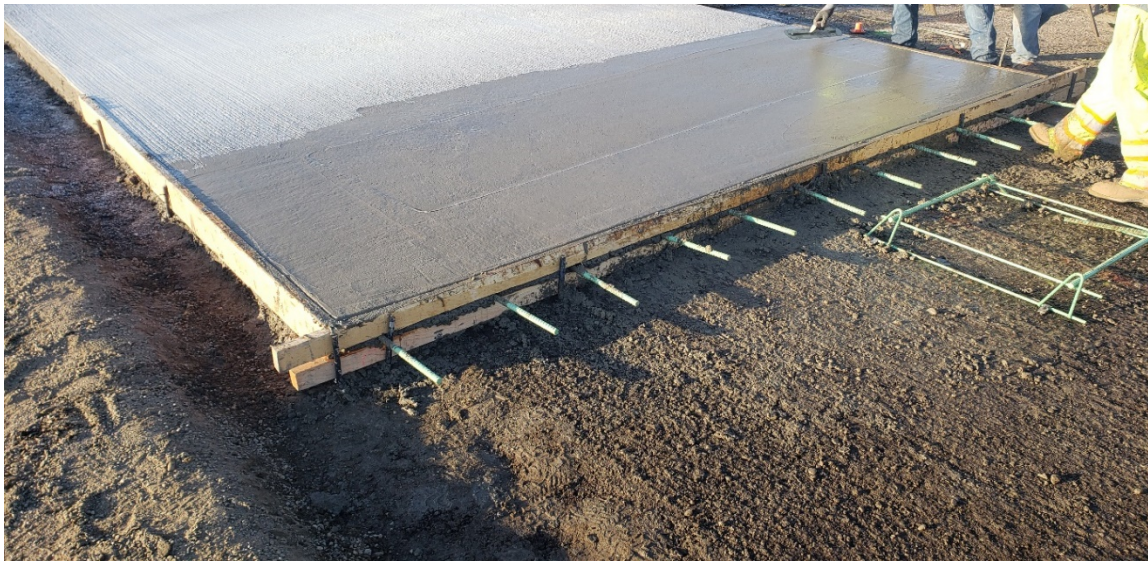
Figure 4.24: Installation of tie bars instead of dowels at a transverse joint (end of paving Shift 1).
