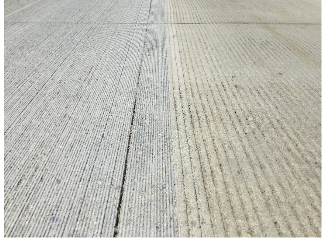
Area on the left side of the photo has been ground; area on the right has not been ground yet (and retains its tined texture)
