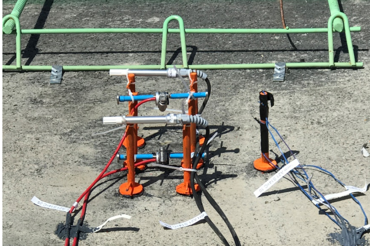
RH sensors (silver sensors with the white cap, back), VWSG (blue, second from back), and thermocouple rod (black, right)
