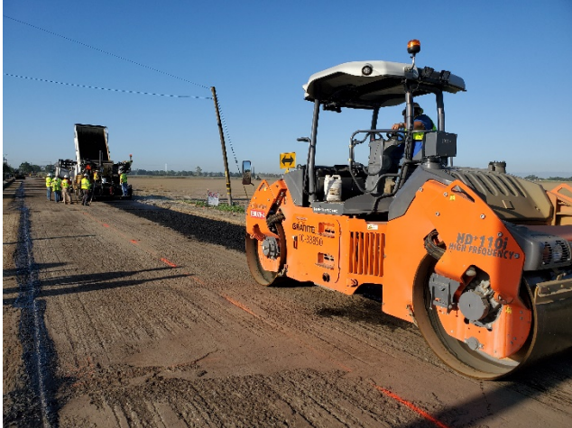
Patching areas with insufficient or missing asphalt base at the shoulder edge of the roadway
