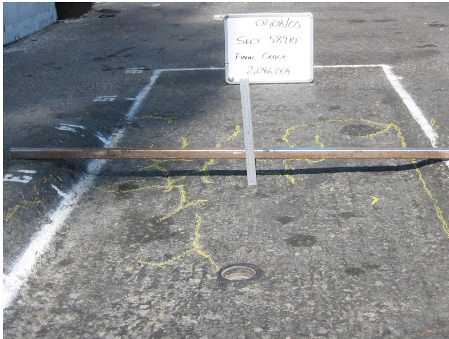
Figure 3.36: Surface cracks marked with crayon between Stations 12 and 14 at end of test.
