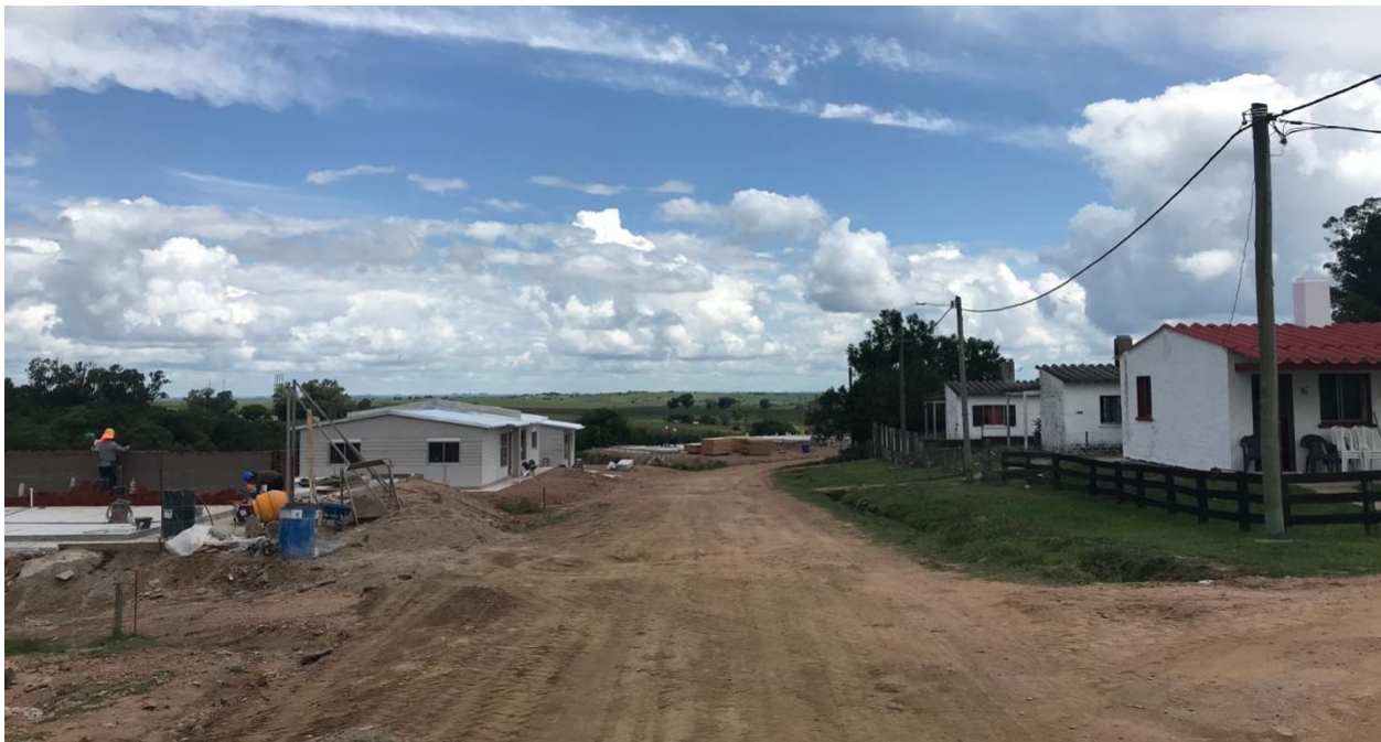
Figure 8: The wood homes, on the left, under construction in Las Flores, Rivera Department, represent a shift from MEVIR’s traditional use of brick, seen in the homes on the right, which were built in the late 1990s (photo by author, 19 January 2024).
