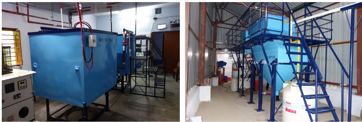
Figure 3: Pictures of the reactor tank and removal tube settler.
