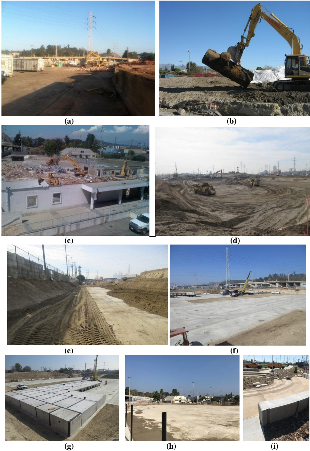
Figure 7. Albion Riverside Park Project photos taken During Construction (a) to (i) (Source: LA Sanitation & Environment).
