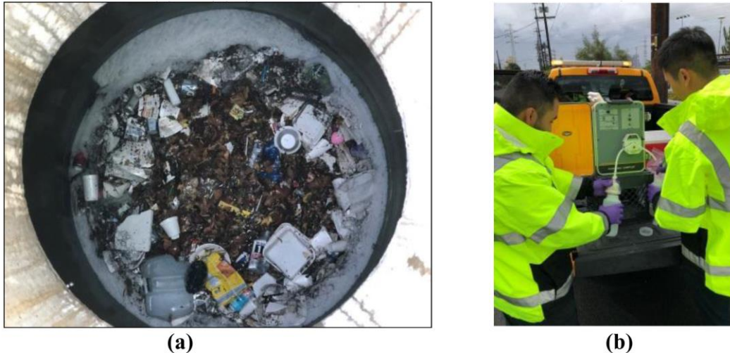
Figure 12. Albion Riverside Park Project Picture of (a) Trash Capture Inside the CDS Unit and (b) Filter of Stormwater to Remove the Settable Solids in the Field on November 20, 2019 (Source: LA Sanitation & Environment).
