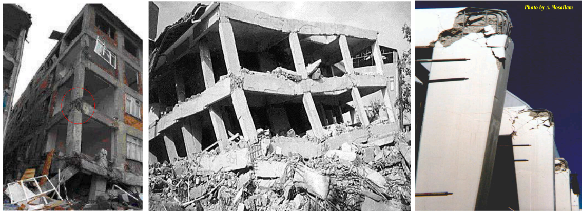
Fig. 1. Examples of damages and collapse of pre-1970s exterior and interior RC beam-column joints during past earthquakes.
