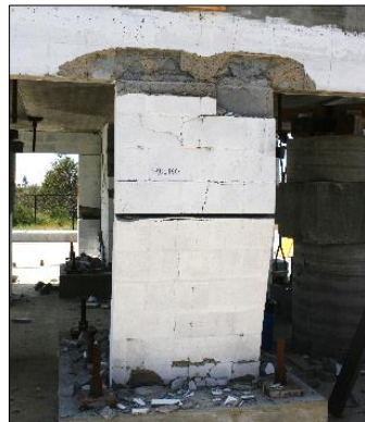
(e) Damage in the flange of Wall-2
