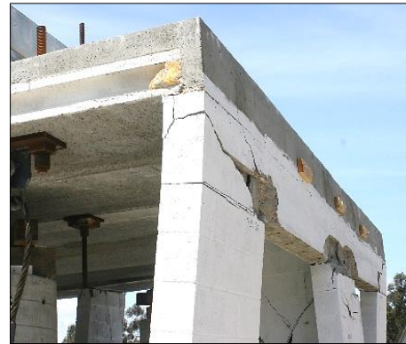
(f) Cracks developed near the roof and the lintels
