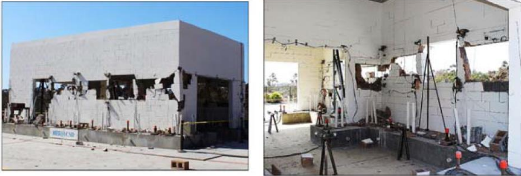
Figure 2-14. Failure of the partially grouted structure tested by Koutras and Shing (2020)
