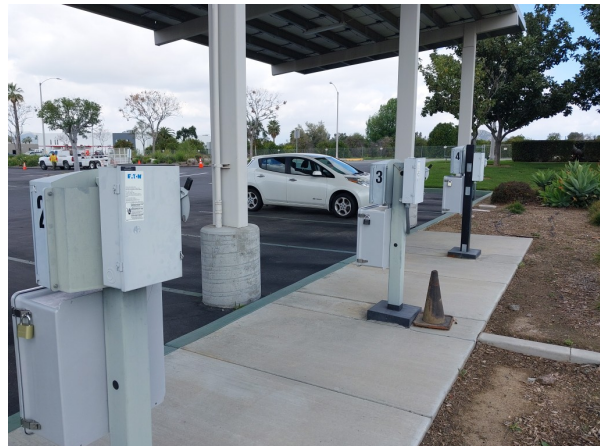
Fig. 5: Level 2 Charging Setup
