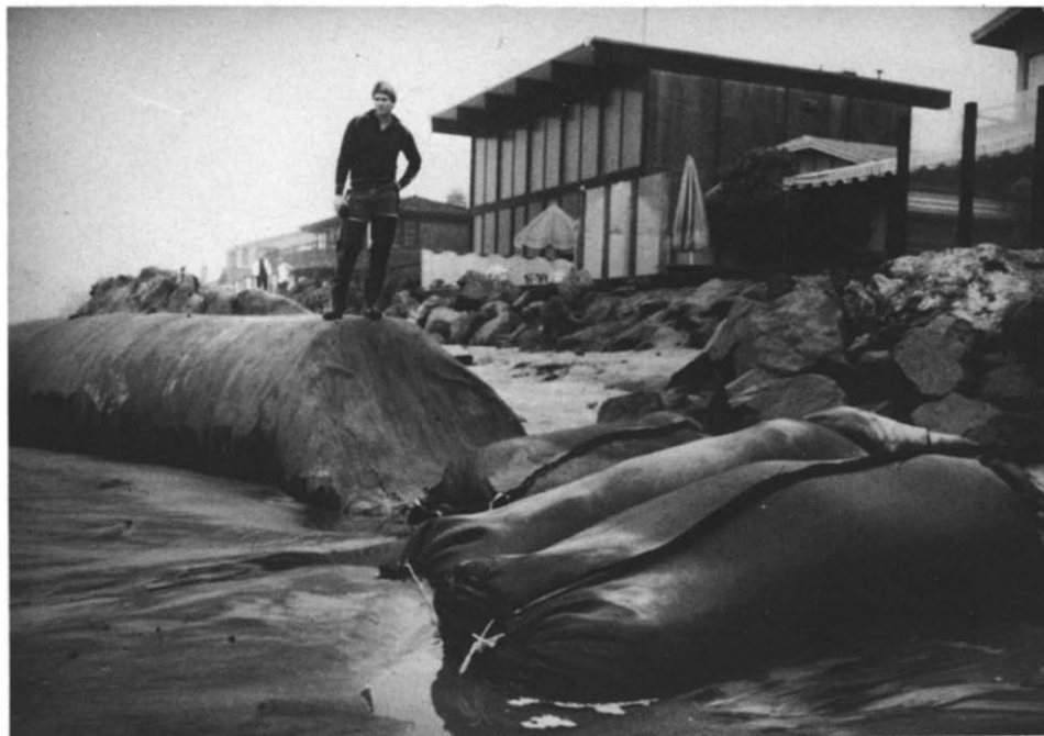
Fig. 3. South end of Longard Tube showing failure of sand-filled bags used as tie-back to effectively hold sand behind the installation during moderate storm of mid January 1981.
