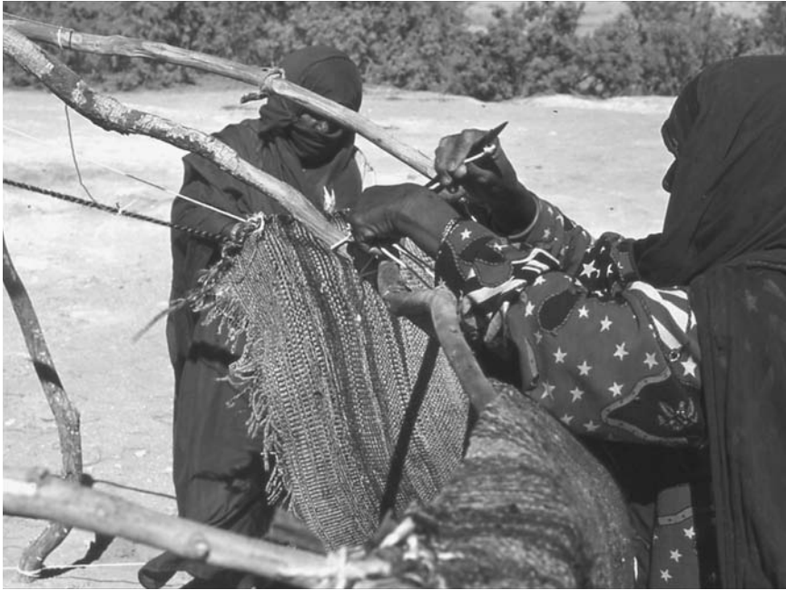
Figure 23.12. Building a beit al-burush : the inner walls of the house consist of tightly woven goat-hair carpets.
