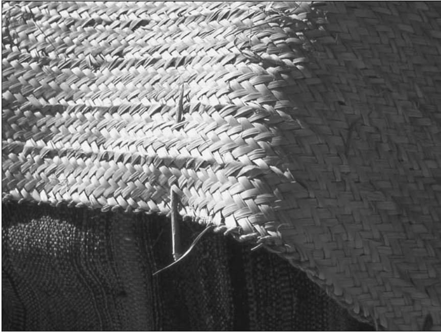
Figure 23.14. Building a beit al-burush : the mats are stitched together with sharp pegs of acacia wood.
