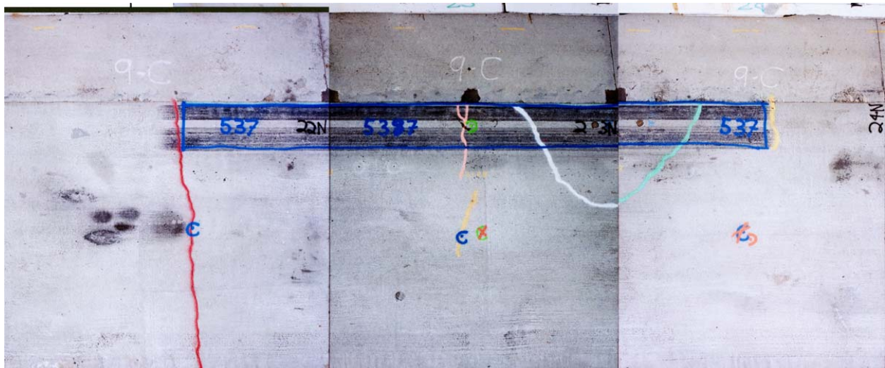
Figure 54. Composite image of Test 537FD showing cracks.
