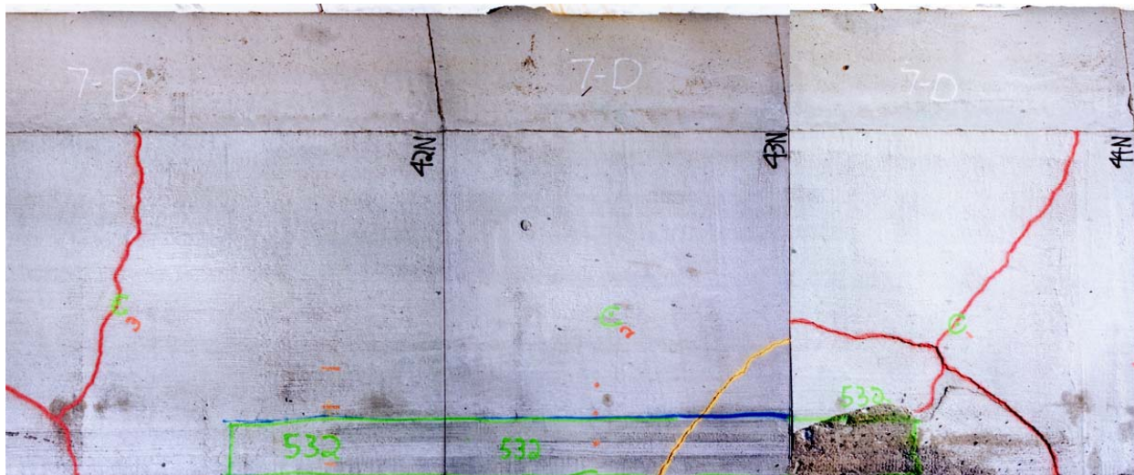
Figure 14. Composite image of Test 532FD showing cracks.
