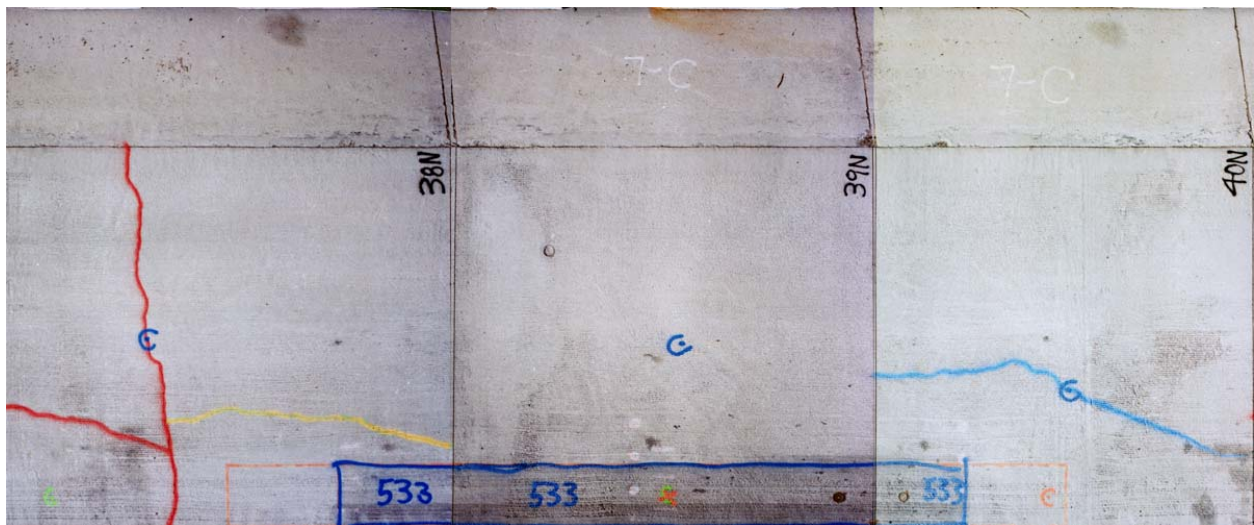
Figure 18. Composite image of Test 533FD showing cracks.
