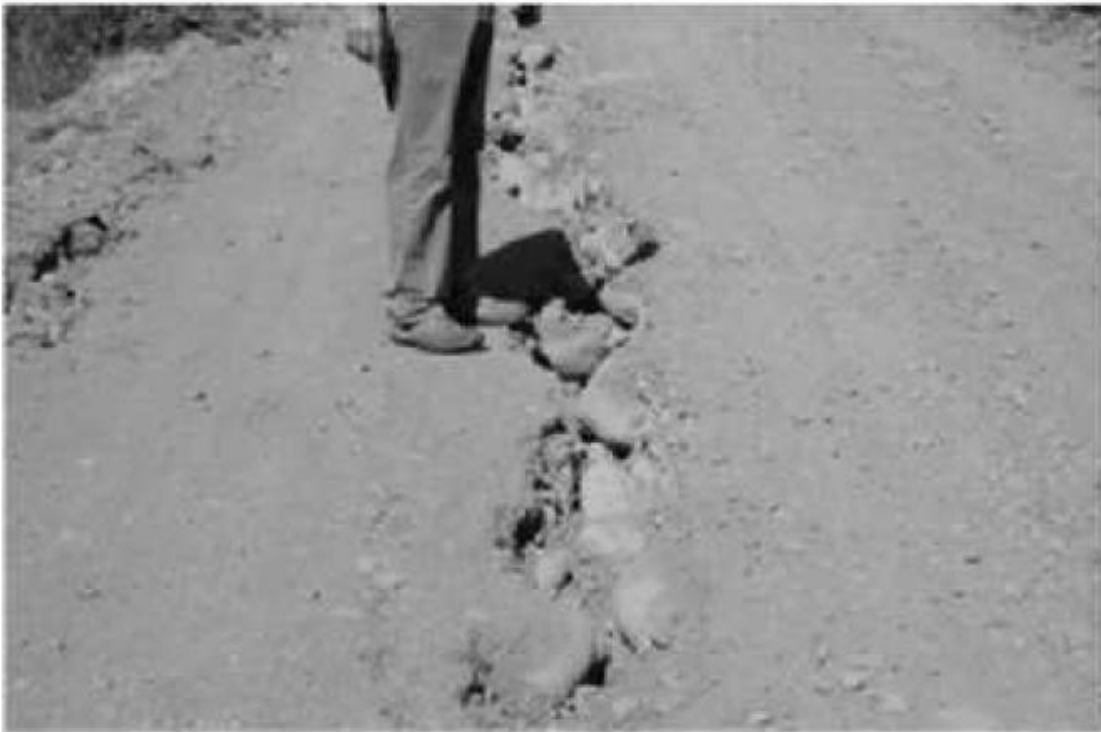
Figure A.7. Top: Failure of the upstream slope of Coihueco dam bottom: Longitudinal crack along crest (Verdugo et al. 2012).
