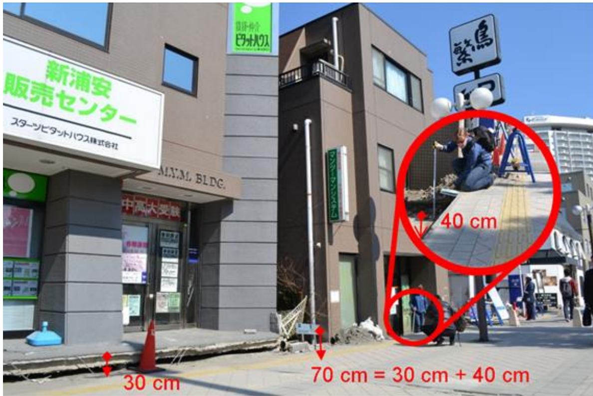
Figure 5.2. Differing responses of pile-supported building (left) and shallow-founded building (right) relative to free-field ground (from Ashford et al. 2011).
