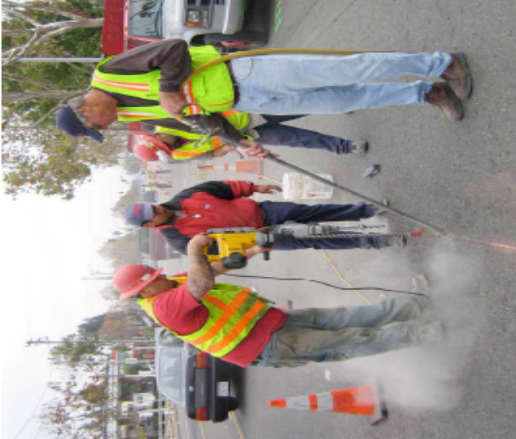
Figure 23 East 14 th Street. Installation: Two Team Installation (Drilling, Cleaning Holes and Placing Magnets)
