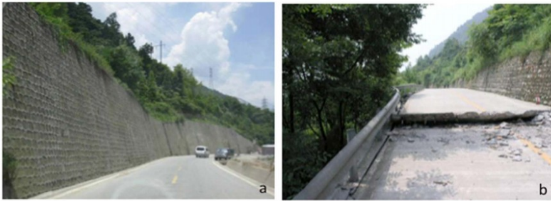
Fig. 2. Conventional retaining structures in the epicentral region of the Wenchuan 2008 Earthquake. Note the fault break in the picture on the right. (Photo: N. Sitar).
