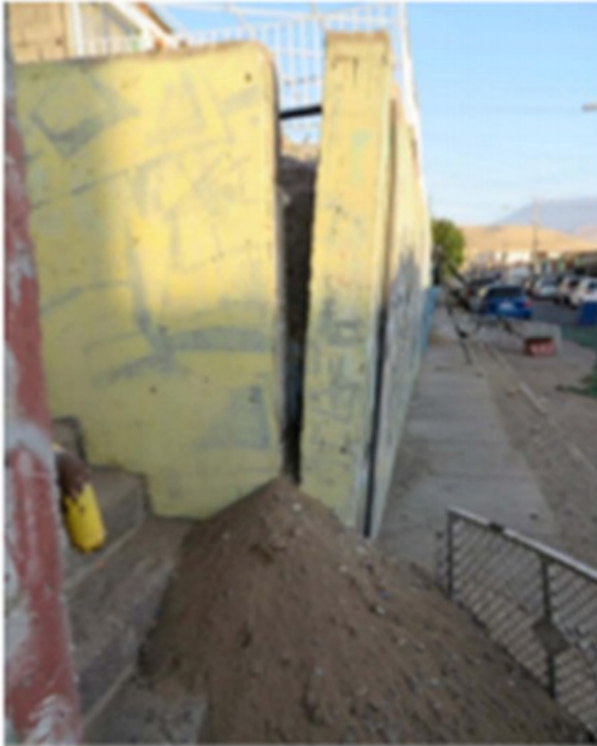
Fig. 3. Reinforced concrete wall without a footing rotated during the 2014 Iquique, Chile, earthquake. (Photo courtesy of G. Candia).
