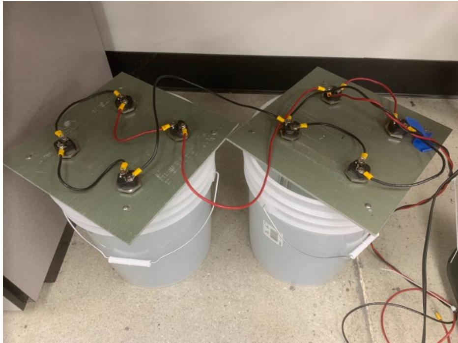
Figure 39. Water Heater Element Resistive Load for Higher Power Test
