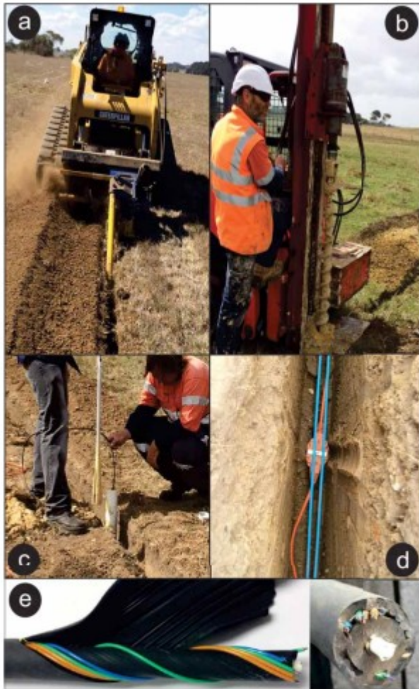
Figure 1. Experimental set-up. (a) Trencher digging the trench, (b) boring for the 4 m deep PVC-cased bores to install geophones, (c) installation of a geophone in a bore and the geophone cables, (d) blue iDAS fibre-optic cables laying at the bottom of each trench, and (e) HW cable buried in the line 5 trench for direct comparison (after Hornman et al. 2013).
