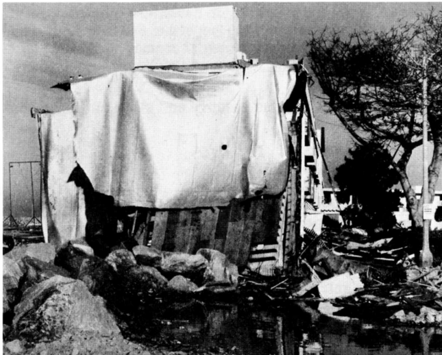
Figure 2. Photo showing collapsed roof section of Portofino Inn, located on Mole B, inside King Harbor, Redondo Beach. Hotel guests were rescued off the roof of the damaged structure by a news helicopter on Sunday evening, 17 January 1988.
