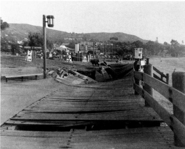
Figure 7. Sections of the main boardwalk at Laguna Beach collapsed after heavy wave surge eroded the sand and undermined piling foundations.
