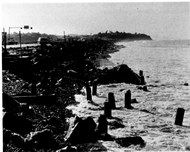
Figure 9. North San Diego County shoreline at Cardiff showing bared cobble and bedrock beach stripped of sand. Old pilings and foundations of previous structures are rarely exposed.
