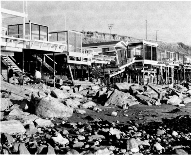
Figure 6. The trailer park at El Morro Beach suffered extensive damage to pipe pilings that support the trailer platforms. The entire cove area was stripped of sand.
