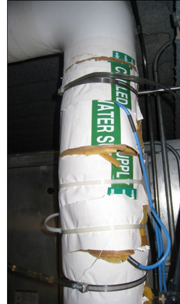
Figure 2.2.1-5d: Chilled water flow and temperature metering
