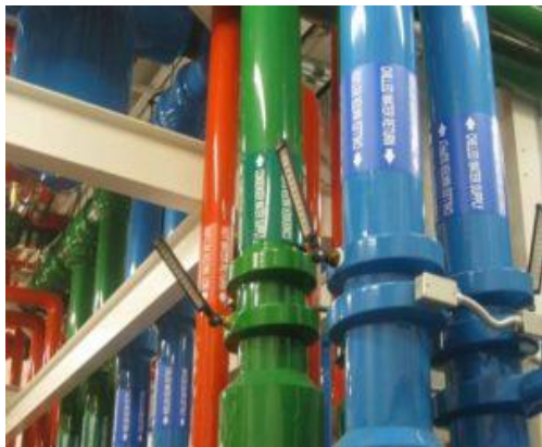
Pipe identified by color (blue: potable cold water, green: hot water, and red: fire water) www.safetysign.com/blog/brimar-is-coming-to-the-ahr-expo/ visited by Briones on 11/02/2017
