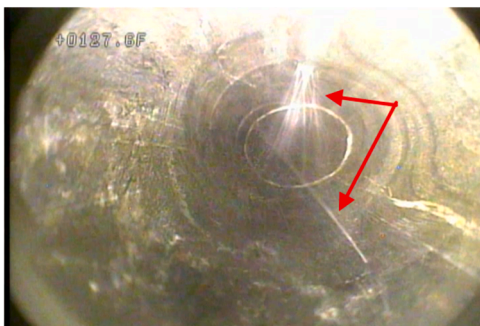
Fig. 4. E1. Water jetting into borehole E1-P (see arrows).
