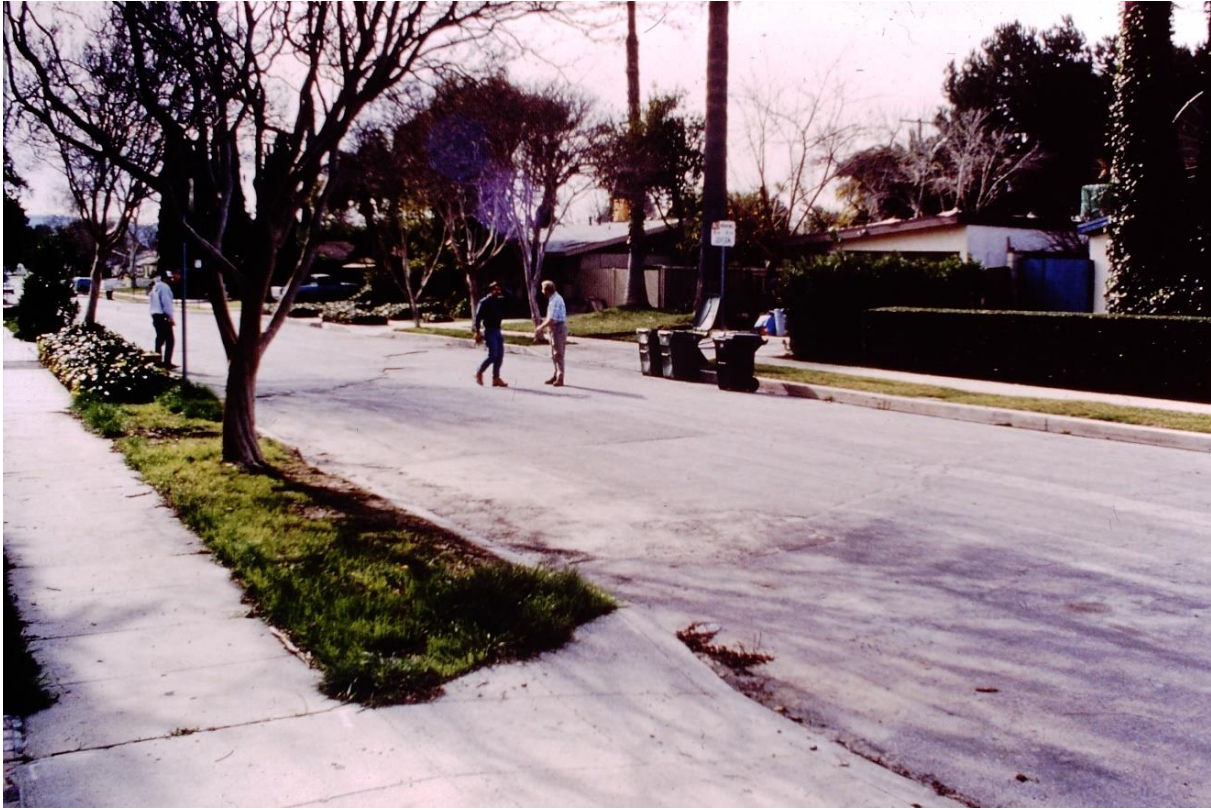
Figure 6.1. Ground cracks and extensional graben deformation along Wynne Avenue, one year after the Northridge earthquake (photograph taken on January 19, 1995 by T. L. Holzer).
