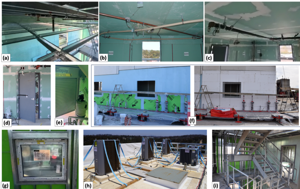
Figure 4. Nonstructural components and systems integrated within the test building: (a) suspended ceilings, (b) flexible and rigid gas piping, (c) fire sprinkler system, (d) swing doors, (e) roll-up door, (f) interior and exterior finishes, (g) windows, (h) roof-mounted mechanical equipment, and (i) prefabricated modular steel stairs.
