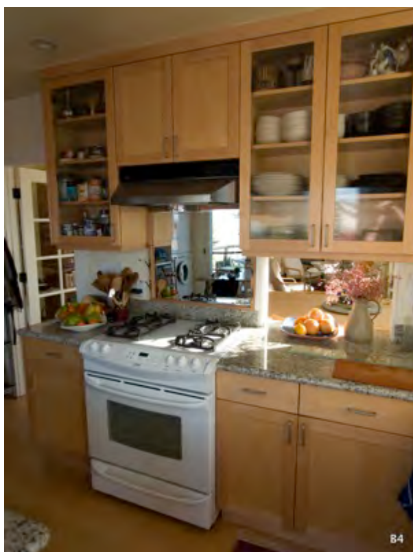
Figure 51. Exhaust System B4; note pass-through behind range.
