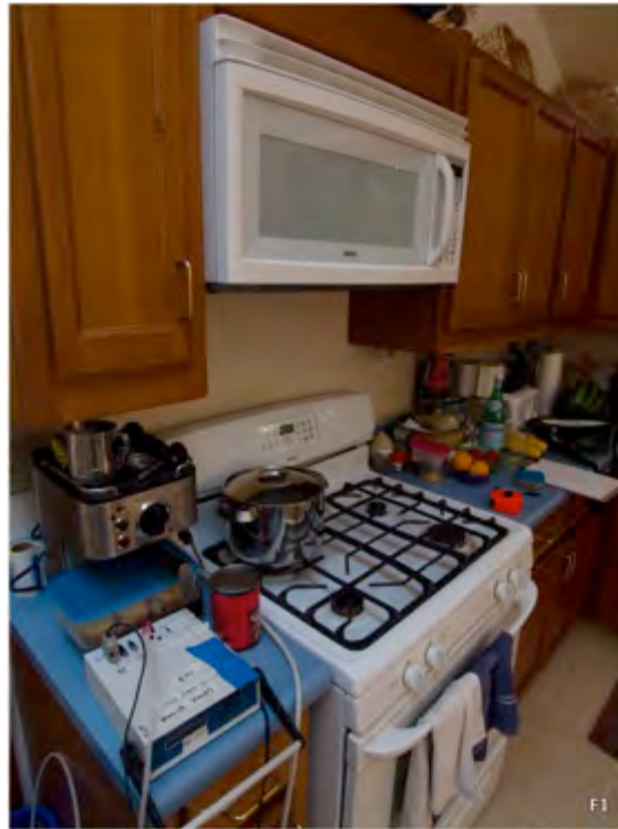
Figure 9. Microwave over range; exhaust system F1, location in kitchen.
