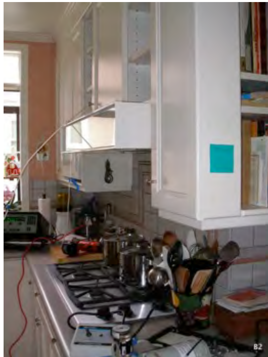
Figure 44. Exhaust System B2; side view showing coverage of cook top.
