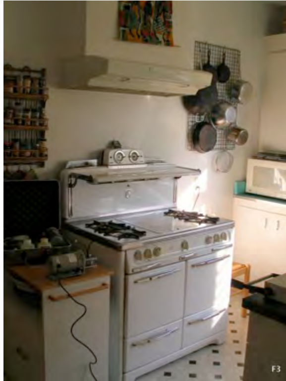
Figure 18. Exhaust system F3, location in kitchen.
