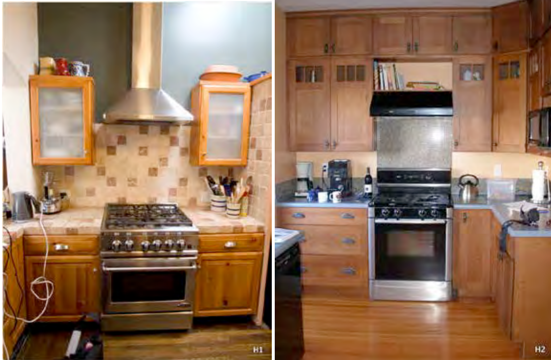
Figure 5. Exhaust hoods with grease screens across bottom opening, H1–H2
