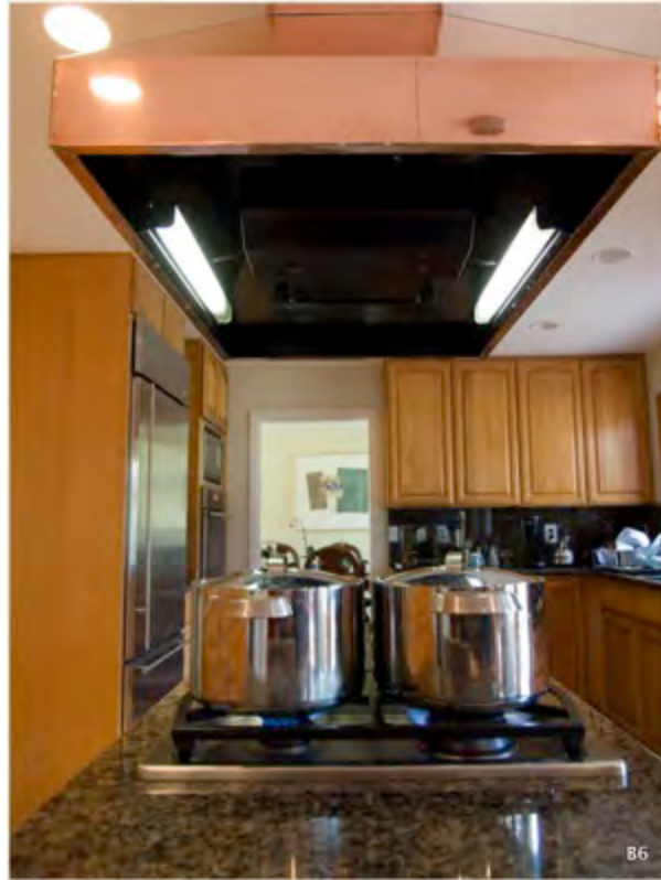
Figure 60. Exhaust System B6; side view showing coverage of cook top.
