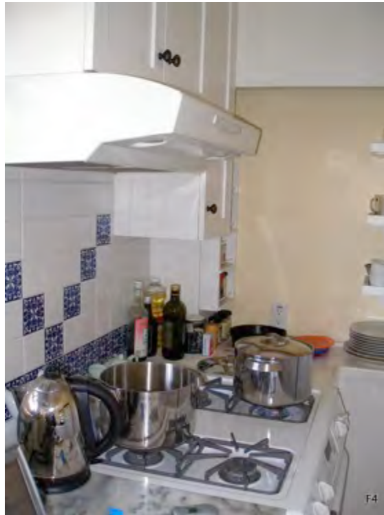
Figure 22. Exhaust system F4, side view.
