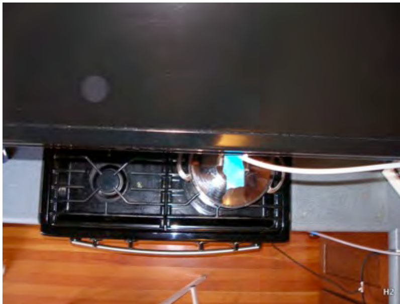
Figure 35. Exhaust System H2; top view showing coverage of cook top.
