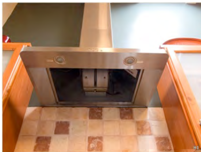
Figure 30. Exhaust System F5 with grease screens removed.
