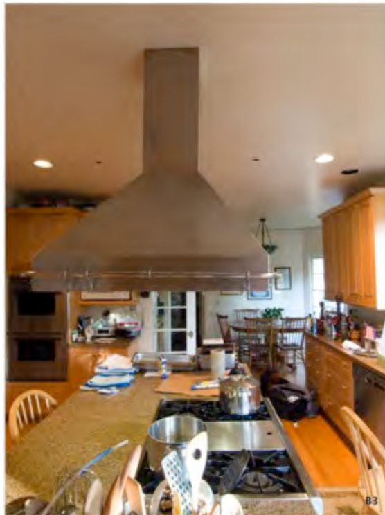
Figure 48. Exhaust System B3; side view showing coverage of cook top.
