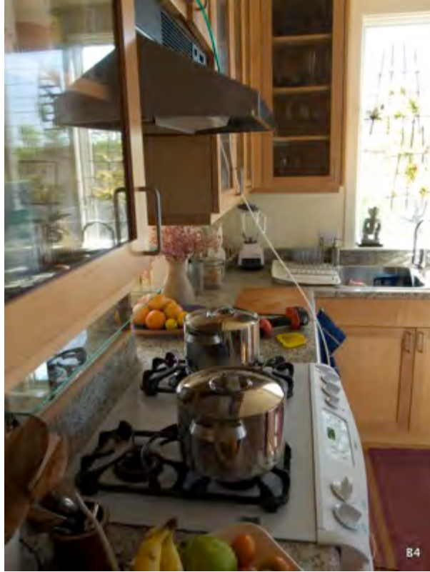
Figure 52. Exhaust System B4; side view showing coverage of cook top.
