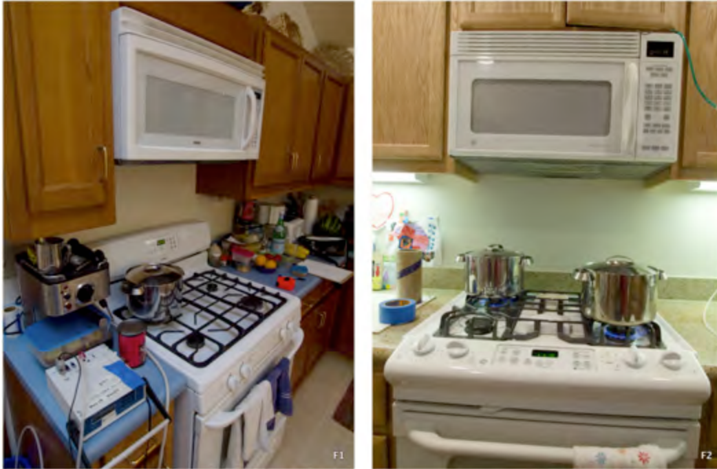
Figure 3. Microwave-over-range exhaust systems F1 and F2
