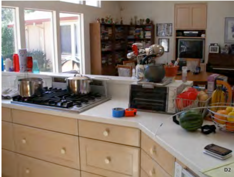
Figure 5. Downdraft exhaust system D2, location in kitchen.
