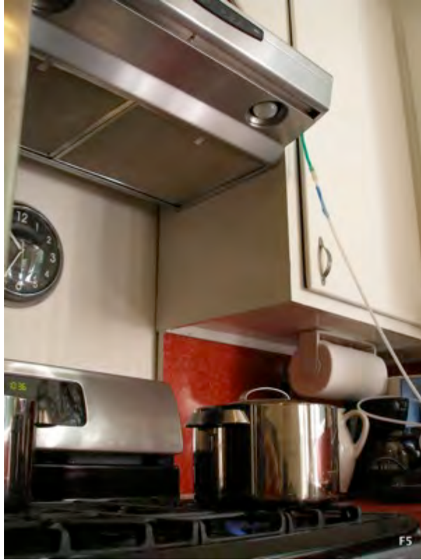
Figure 26. Exhaust System F5 showing profile at bottom.
