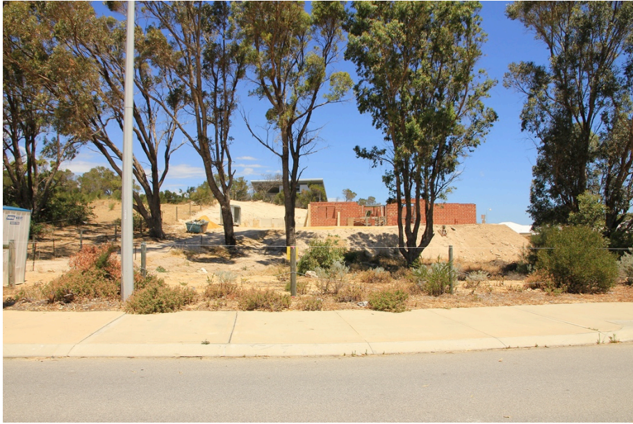
Figure 13. Case 1 (Hartford Grove): view of topographic disturbance caused by cut and fill for concrete slab construction (Author 2013).
