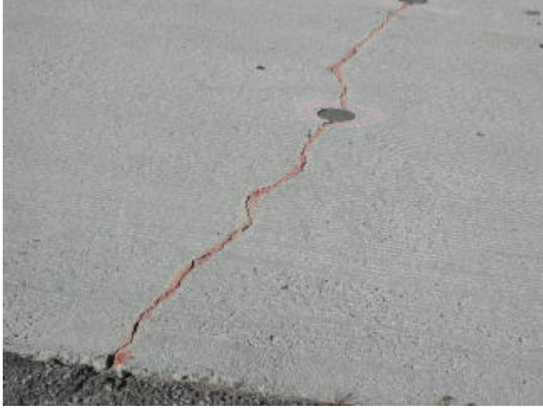
Figure 2.1: Typical early-age thermal cracking of the concrete pavement [1].
