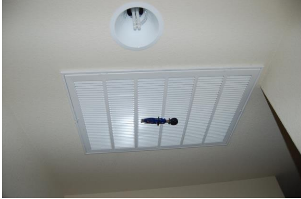
Figure 4 Methods used to monitor central forced air system use: power meter on the air handler (upper left), temperature/relative humidity sensor at the supply grill closest to the air handler (upper right), digital anemometer at the return grill (lower).
