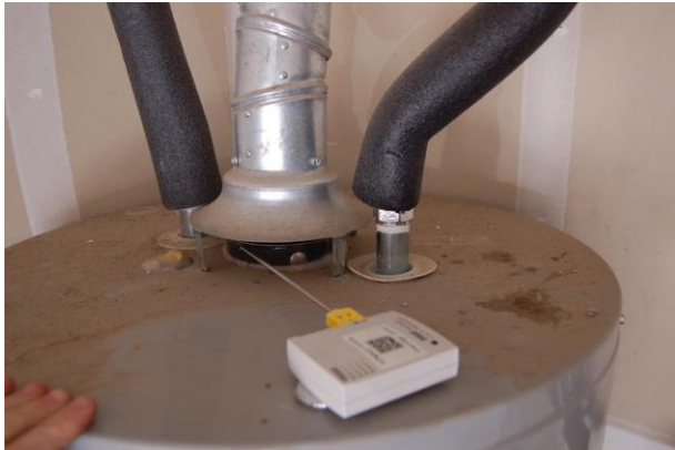
Figure 5 Thermocouple probe used to monitor gas water heater usage.
