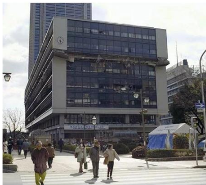
(a) Mid-story collapse in the 6th floor
