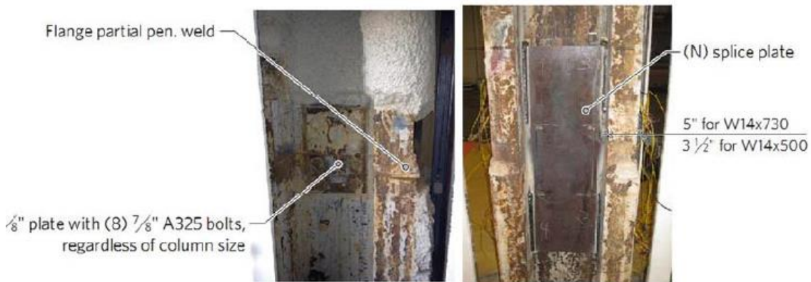
(b) Fix column splices with added plates: before retrofit (left) and after retrofit (right)
