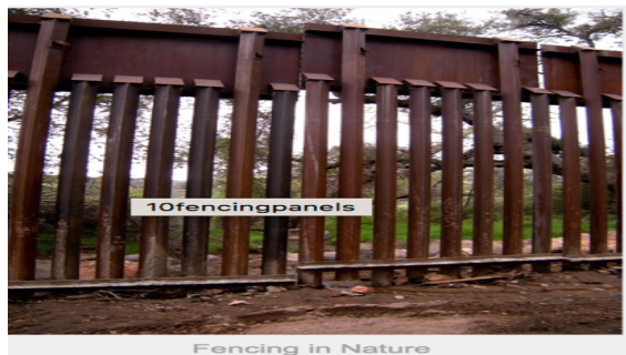
Figure 13 Image taken by the hikers demonstrates how the wall contributes to ecological damages.
